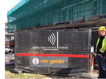
Innovative noise control barriers, placed alongside a water pump
